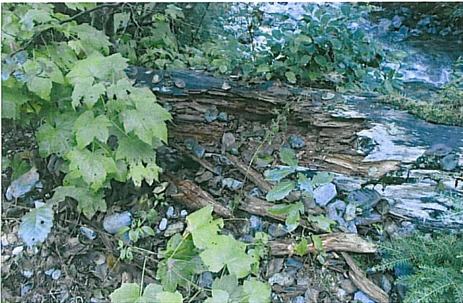
CK-2346 Guard log rotten
